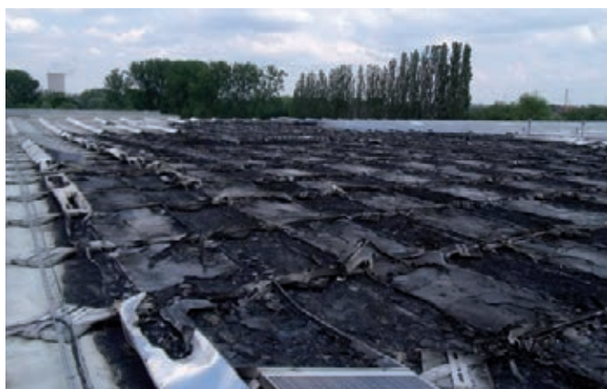
Area of roof after damaging event
